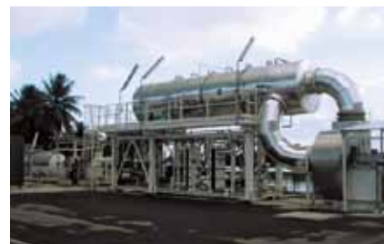
Vapour Compressor in a seawater desalination plant
